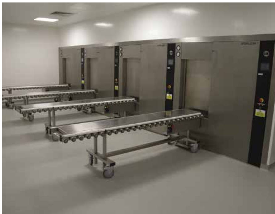
The LTE Scientific 42cu ft sterilisers were sized to suit the width of the building
